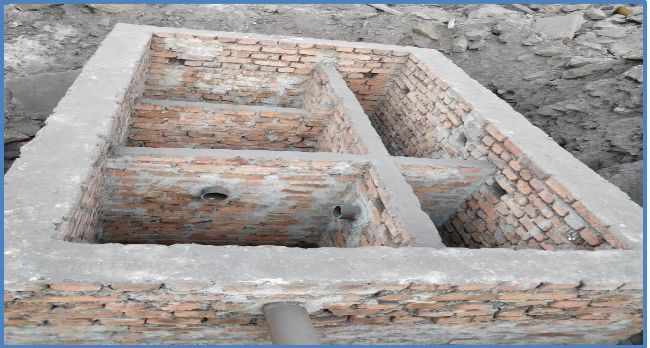
Picture 10 – Oil & Grease Trap
