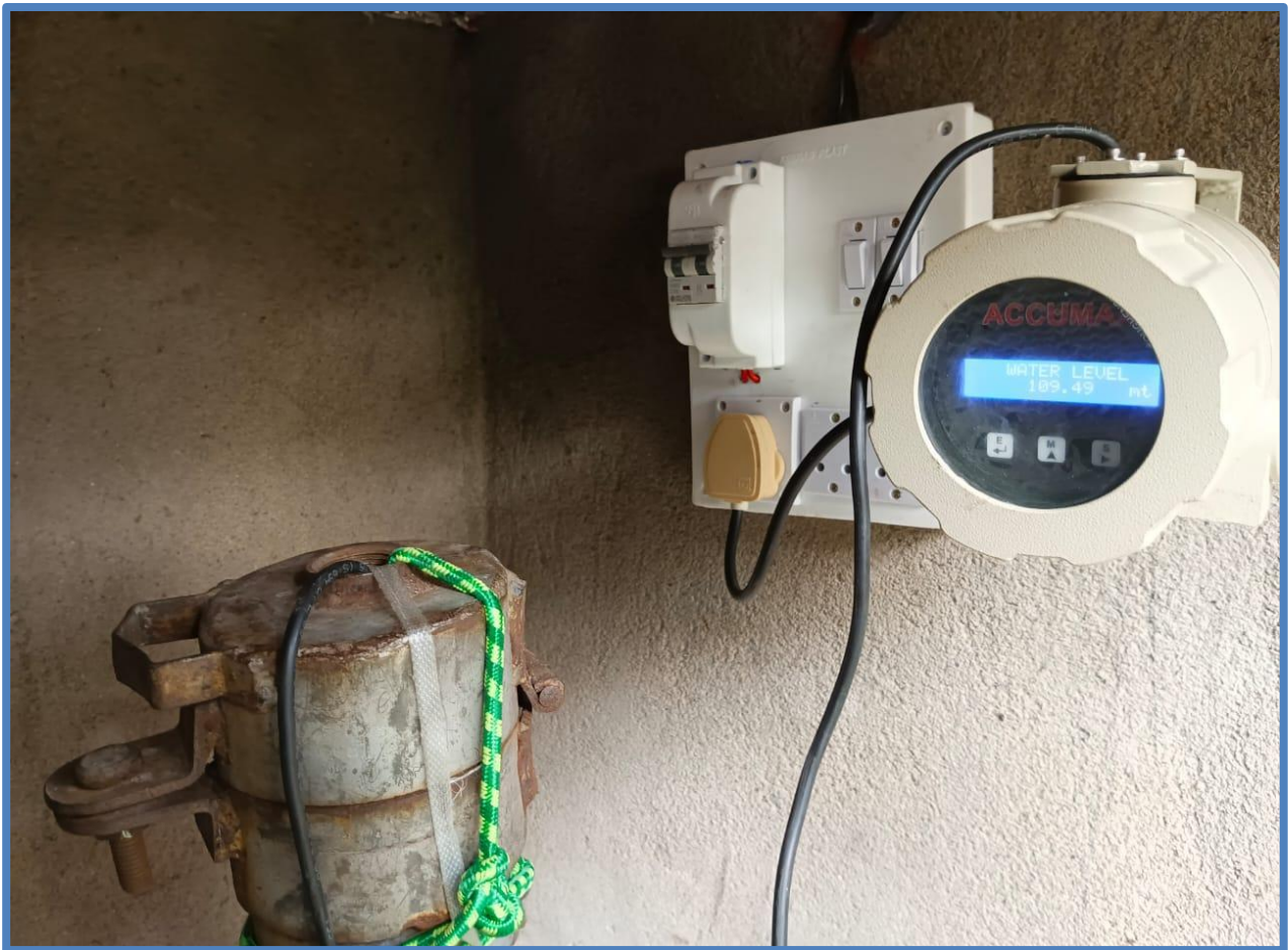
Picture 12 – Piezometer well
