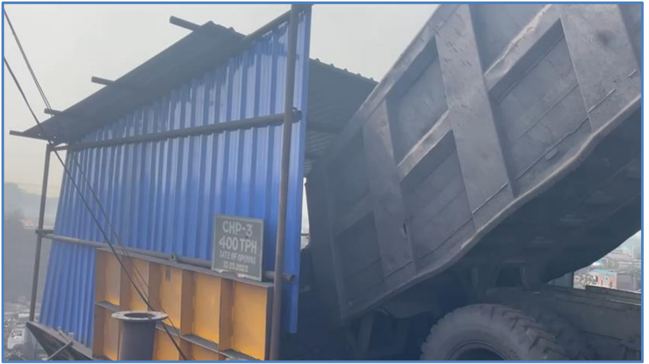
Picture 7 – Enclosed Coal Handling Plant
